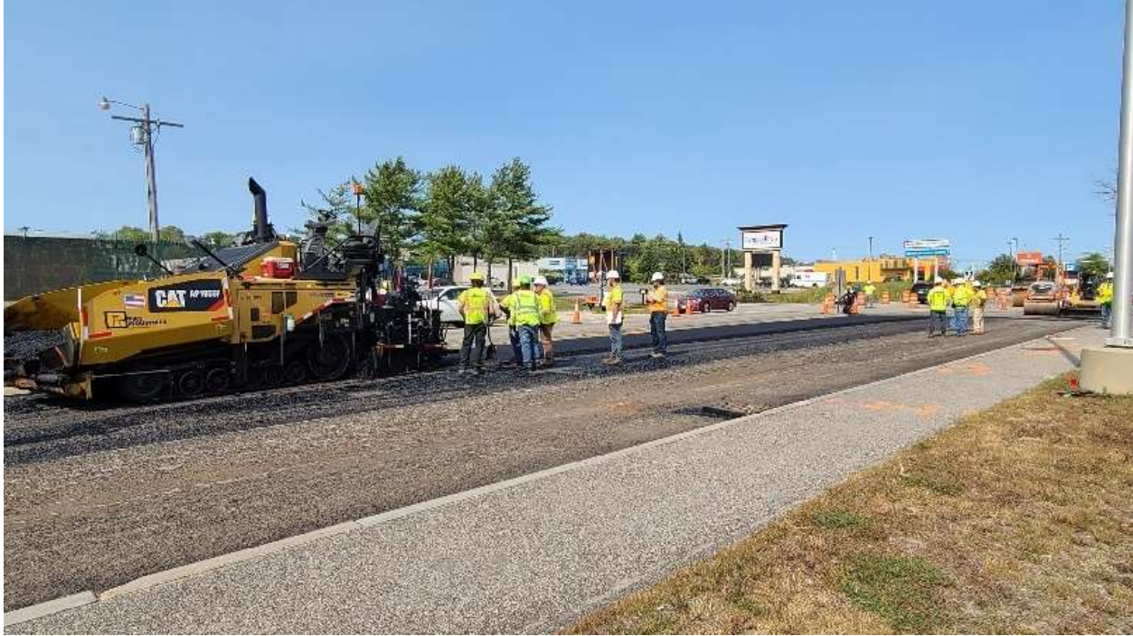
Maine Mall Road being repaved with a new open graded friction course.
